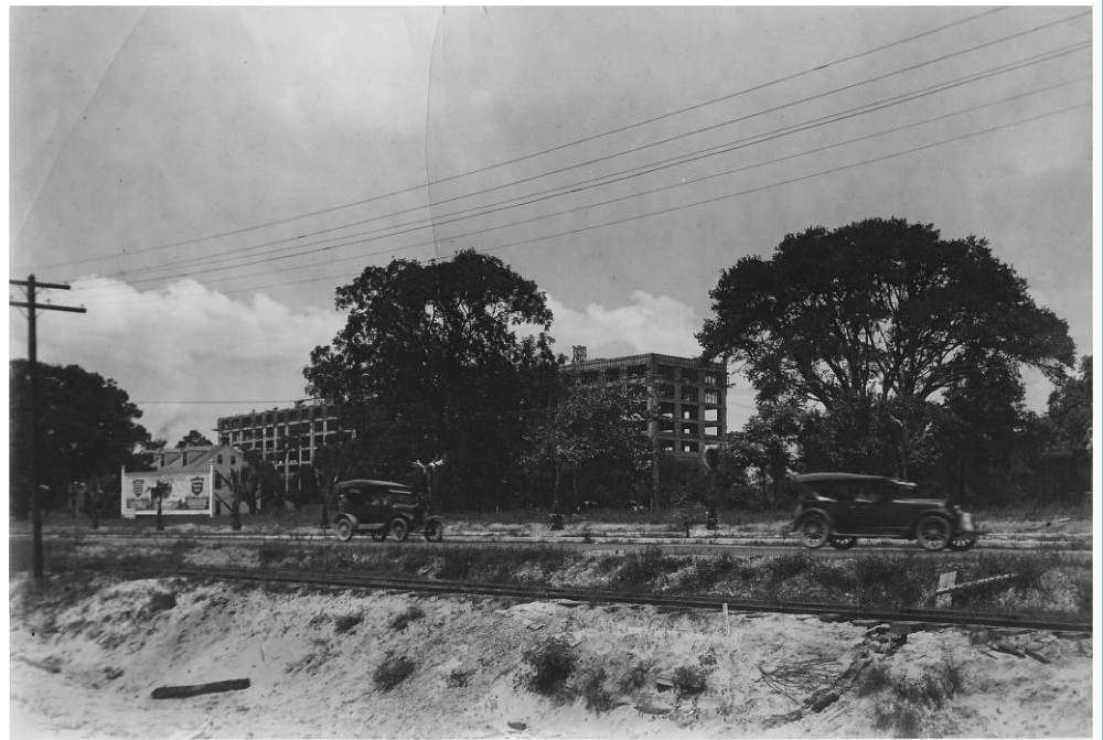
Edgewater Gulf Hotel under construction, 1926... trolley tracks in foreground were no longer in use, Biloxi (Thanks to Randy Randazzo)
