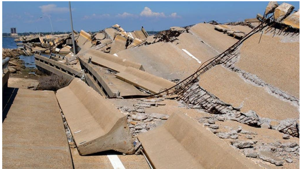
Damage from Hurricane Katrina to the Biloxi-Ocean Springs Bridge presented a monumental construction project, 2005. (Clarion Ledger)
