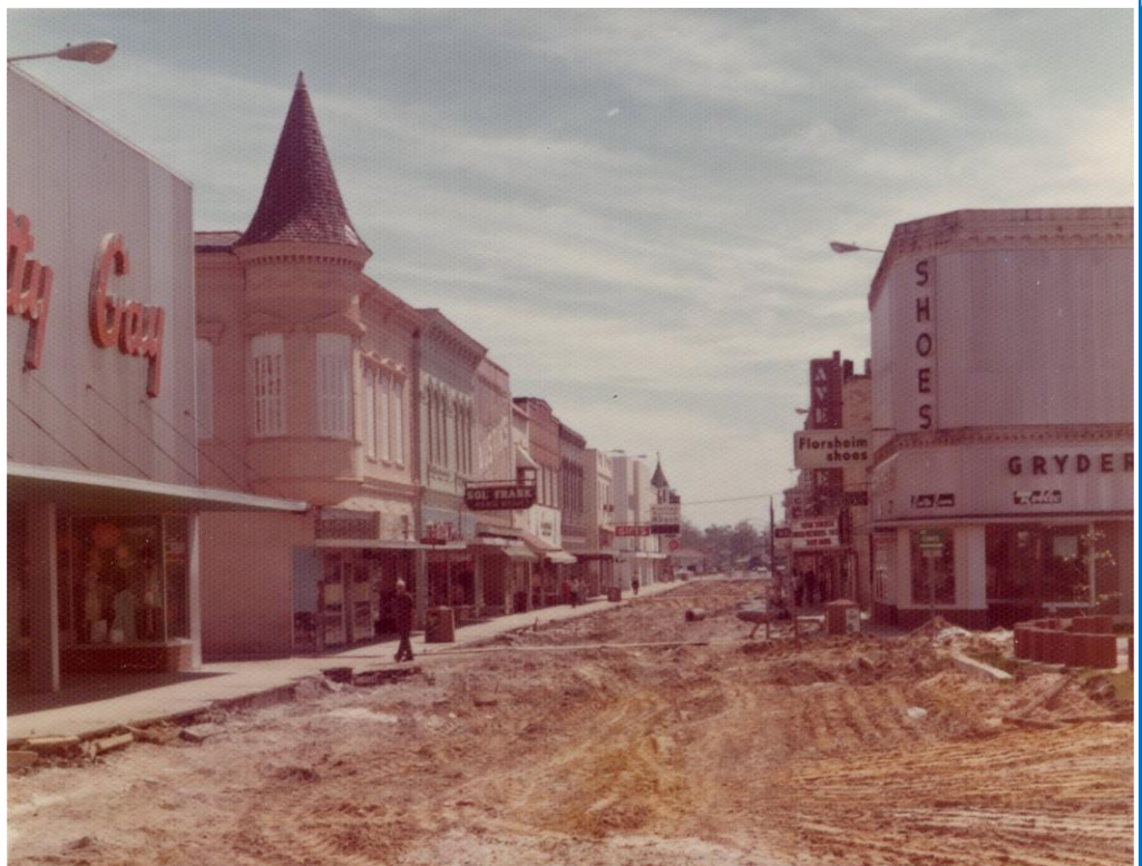
Construction of the Vieux Marche, downtown Howard Avenue, 1976, during urban renewal; Howard Avenue, looking to the east. (Biloxi Library)
