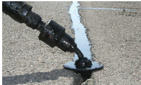
Cracks should be sealed as soon as they are observed.
