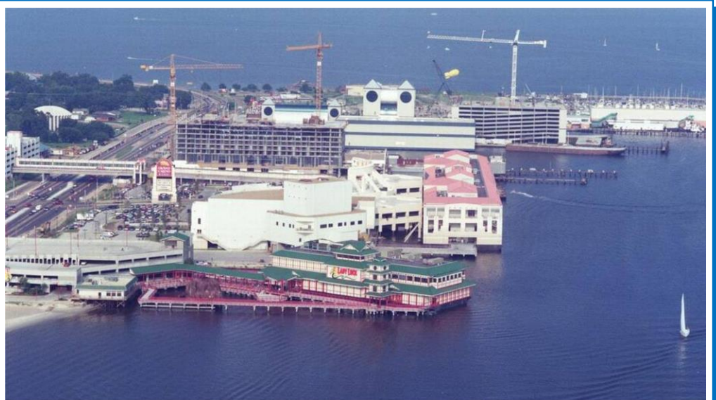
"Casino Row" under construction, Point Cadet, Biloxi, mid-1990s. Lady Luck casino in the front, Casino Magic hotel under construction, cranes in the background at work on Golden Nugget casino.
