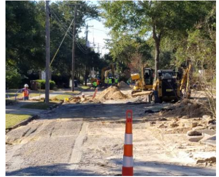
Father Ryan Avenue Infrastructure/FEMA repair project is progressing south of the railroad.
